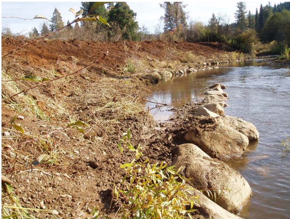
Immediate Post-construction Streambank Treatment Boulder Vanes, Floodplain Bench & Sloped Streambank ( looking upstream from bottom of project )
