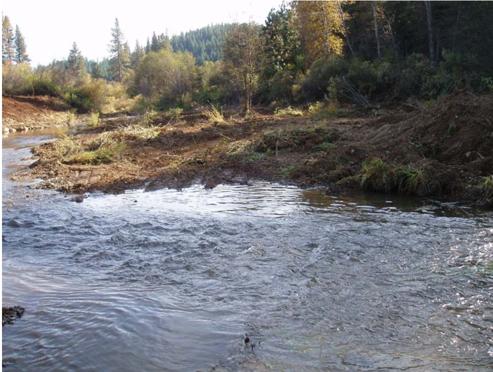
Immediate Post-construction Floodplain and Vegetation Transplants Floodplain Lowered Three-Foot (looking upstream from bottom of project)
