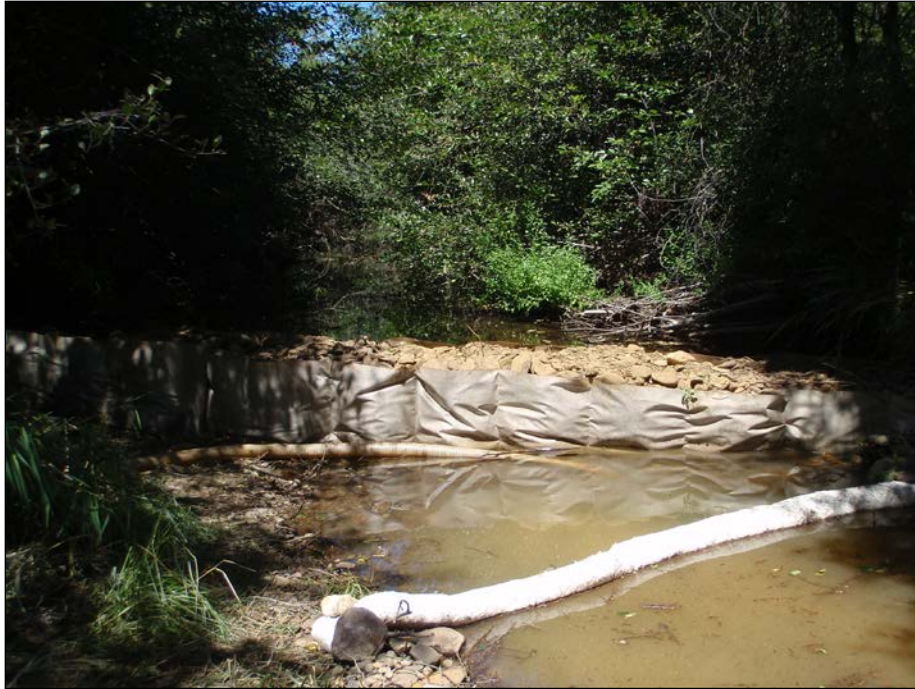
Sediment water quality control dam below construction of fish passage structure at Reid Dam.
